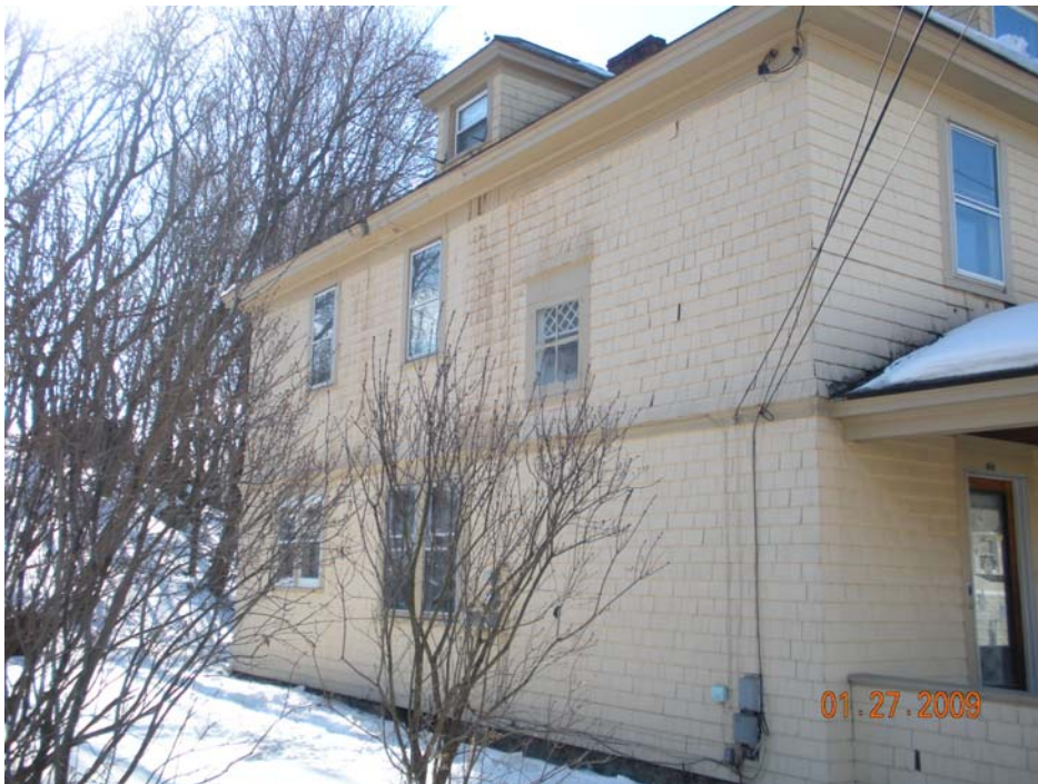
“A” and “B” sides: above porch roof, side wall and “B” side eaves
